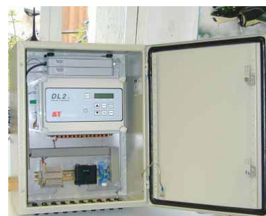
DL2e Logger, GSM modem and antenna, 12V wiring kit and relay, solar power regulator and LBK1 rechargeable battery pack, installed in Weatherproof Enclosure
